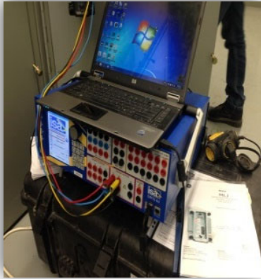
Three Phase Secondary Injection
