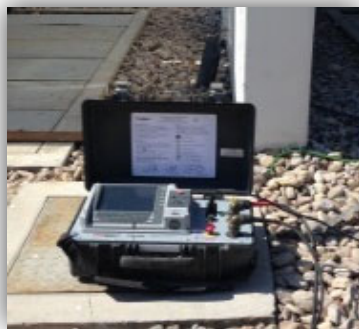
Three Phase Transformer Ratio Test
