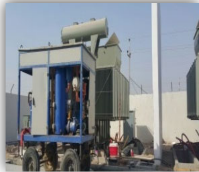
Transformer Oil Purification
